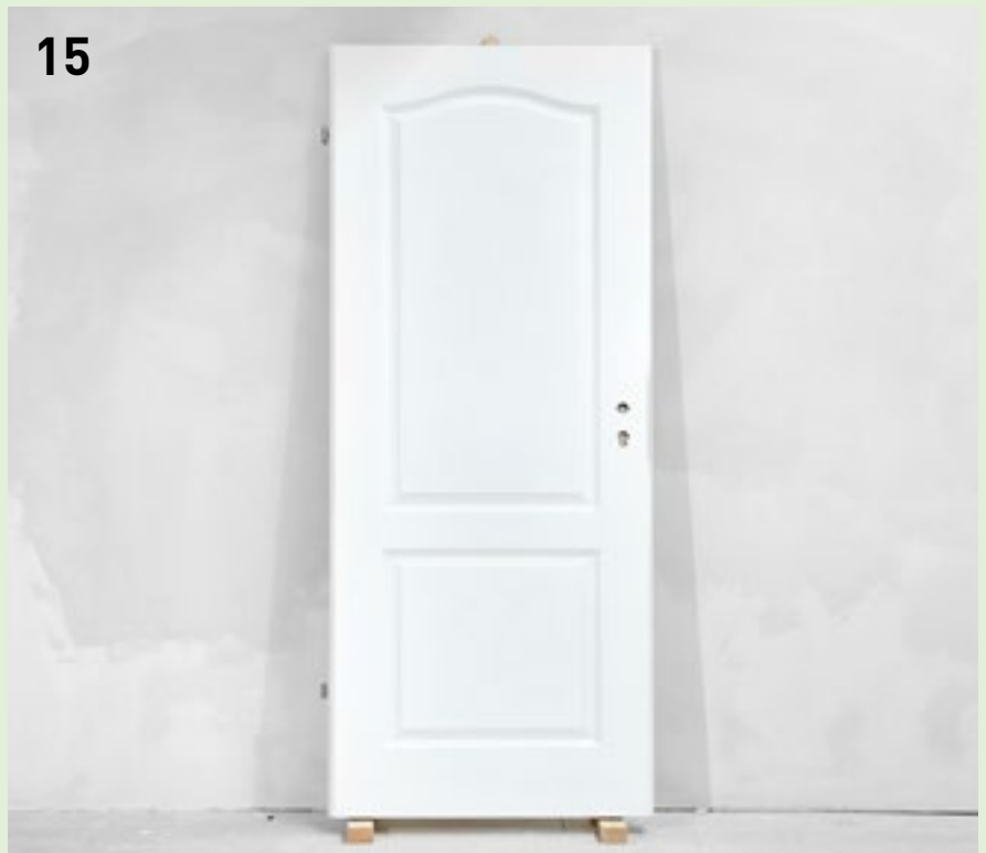
Done! But only when the paint is well and truly dried through is the painter really finished. At that point, the door fixtures can be attached and the door can be rehung.
