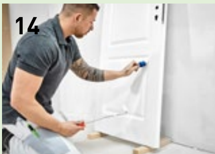
Apply a final coat using a brush (profiles) and roller (surfaces); multiple coats may be necessary.
