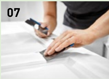
After stripping the old paint, smooth out uneven and damaged areas and fill small holes.
