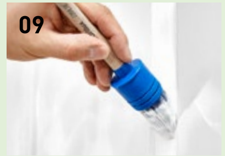
Apply primer to the surfaces using a roller and to the profiles using a brush and then let it dry thoroughly (observe drying time specified by the manufacturer).
